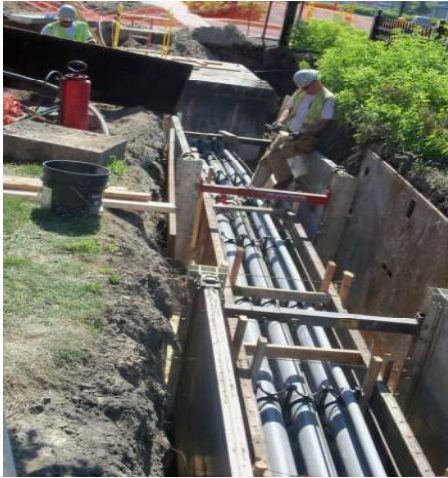
Utility installation at University of Minnesota Biomedical Discovery District Cardio Cancer Building
